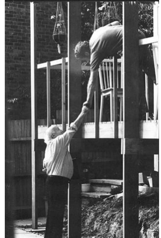
Figure 4. Walter and Ken, working together on one of the self-built houses in the Lewisham housing scheme.
